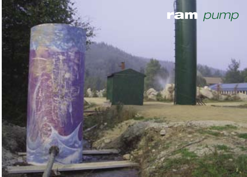
The supply tank situated in the creek, with the geothermal well house and storage tank in the background.
