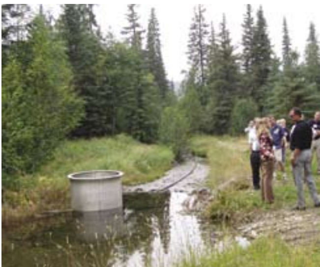
Gwen at the dam site, with the partially buried stainless steel inlet.
